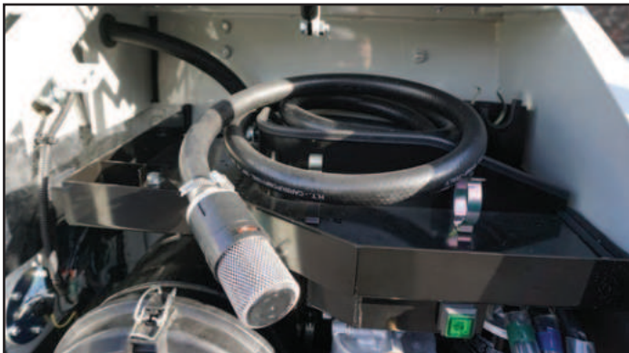
Fuel Transfer Pump
